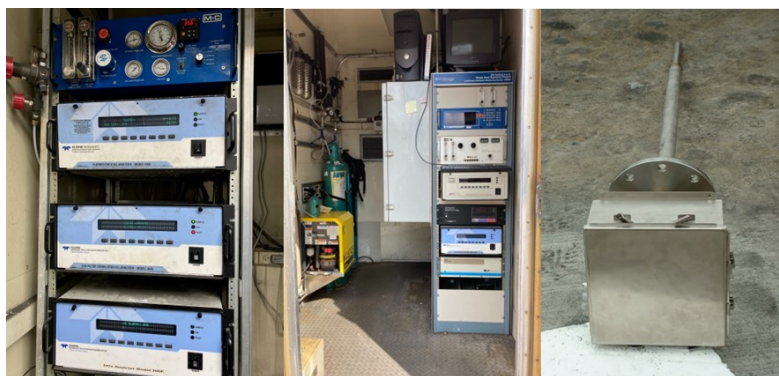
Figure 1. Left: CEMS analysers, Middle: CEMS room, Right: stack probe.
